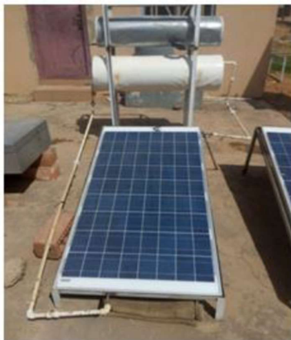
PV with cooling system
